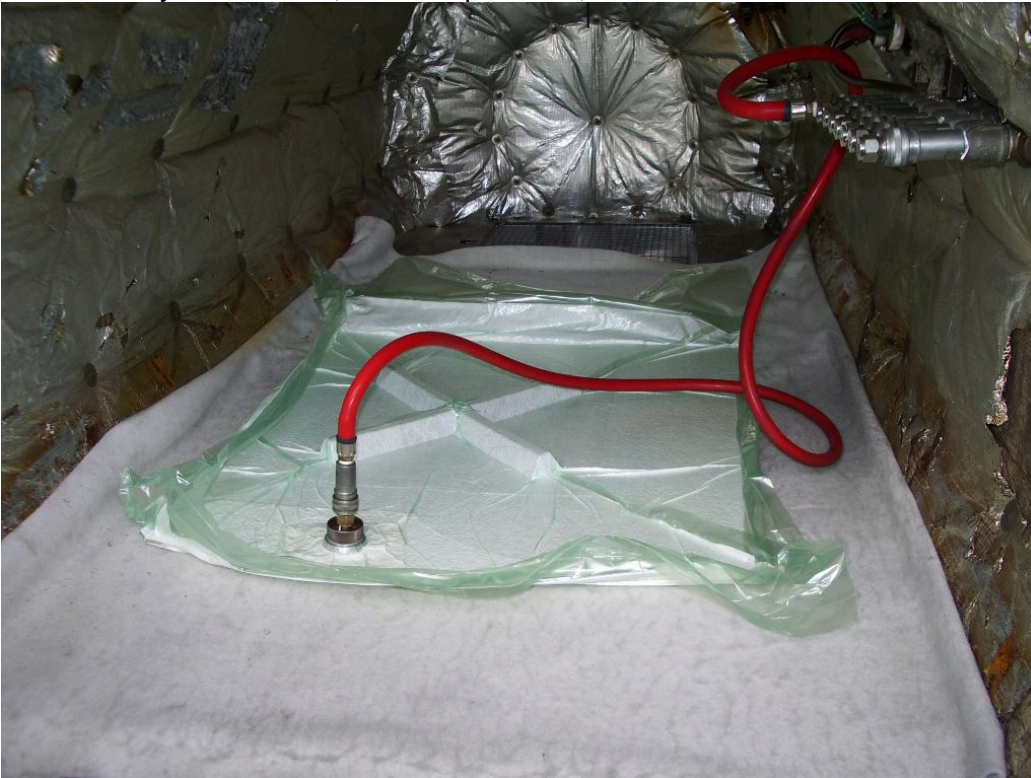
Autoclave Cycle at 120°C, 4bars of pressure, duration 2h
